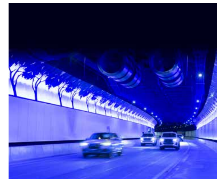
Figure 65. NorthConnex, Sydney. Australia's first "feature lighting tunnel" demonstrates enhanced visual amenity to users.
